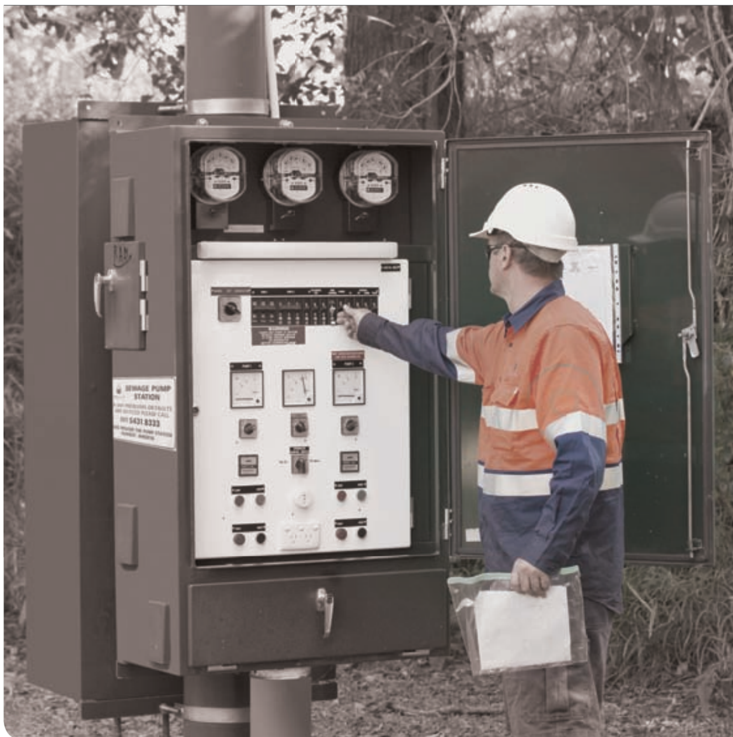
Rod | Sewage Pump Station — Bli Bli, 5.30am
