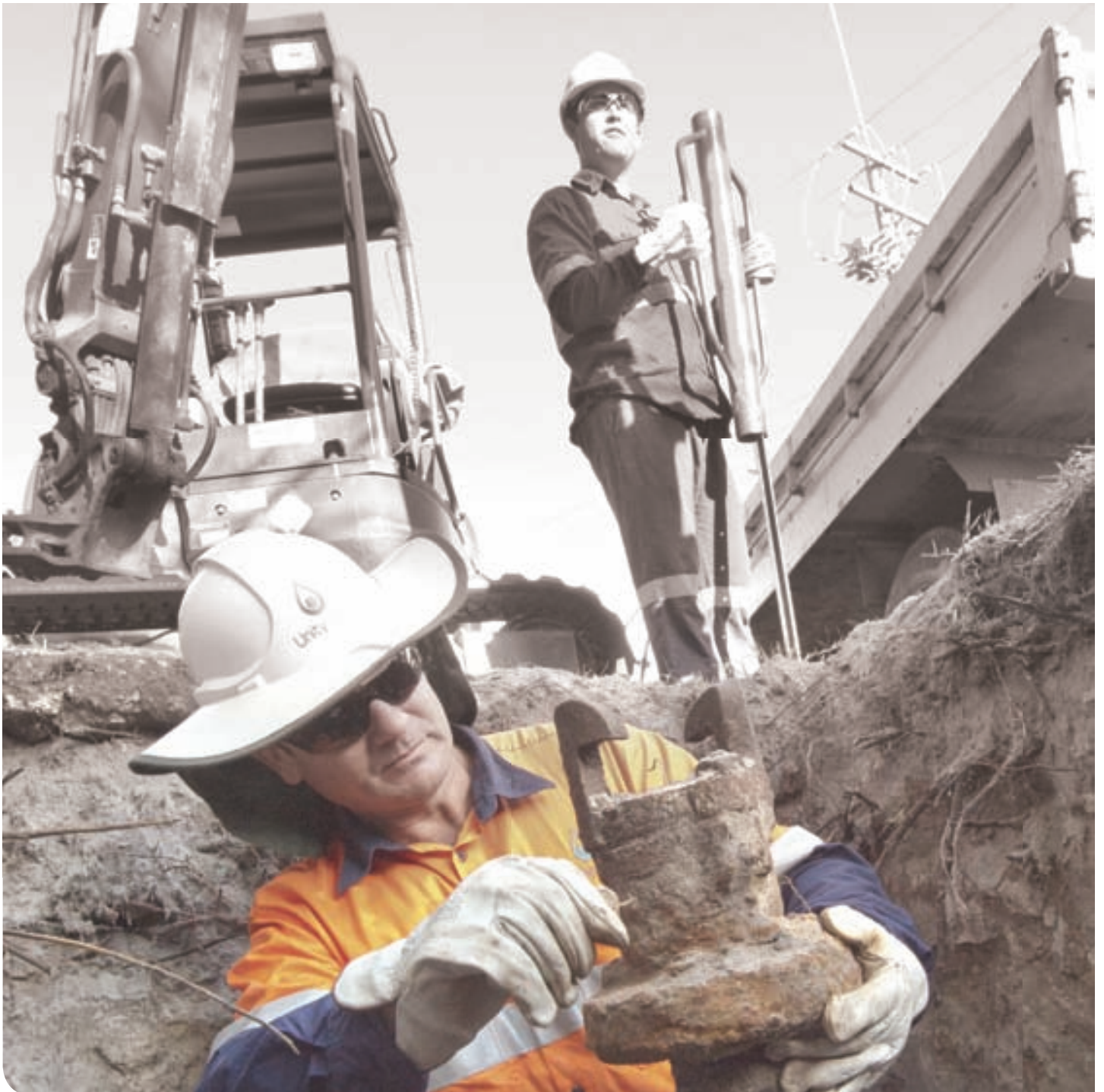
Arron and Brock | Field workers replacing valves to improve reliability and quality of water delivered to your home — Redcliffe 11am
